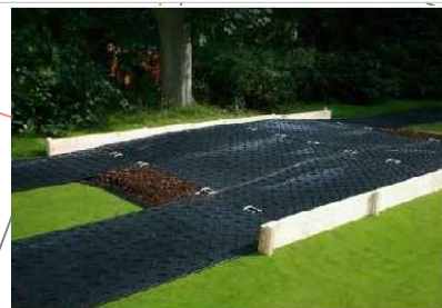
Ground Guard trackways should have additional cushioning installed where they pass near to trees.
